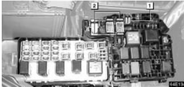
► Engine compartment 1 Pull-out tool 2 Spare fuses
