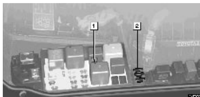
► Engine compartment 1 Pull-out tool 2 Spare fuses
